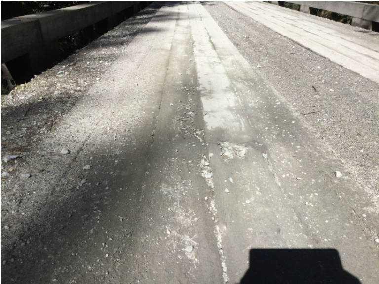
Wear plank condition
