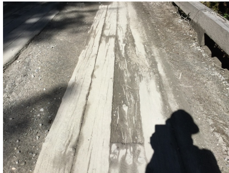
Wear plank condition
